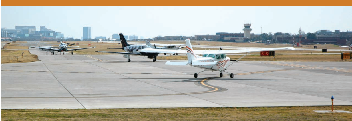
At Addison Airport, two new concrete aircraft holding bays were constructed on both ends of Taxiway Alpha. The north aircraft holding bay capacity was increased by 35 percent compared to the existing holding bay configuration.
